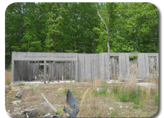
Poorly maintained vacant structure
