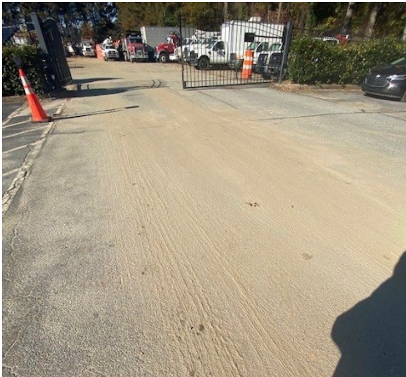
Dirt observed at the front of the site, carried from the rear unpaved area
