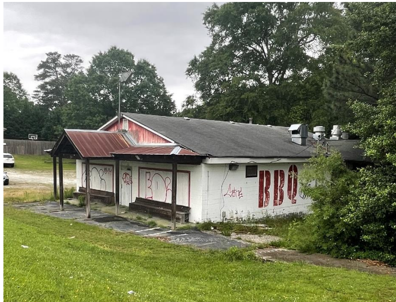
Vacant Commercial Structure at 2662 Loganville Highway
