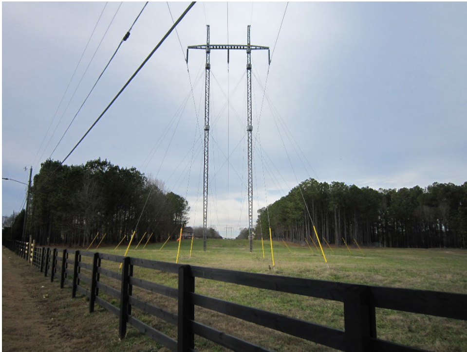
View of overhead power lines where multi-use path is required underneath
