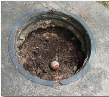
Storm drain full of yard debris and other trash
