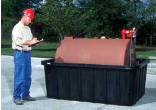
Temporary secondary containment without cover
