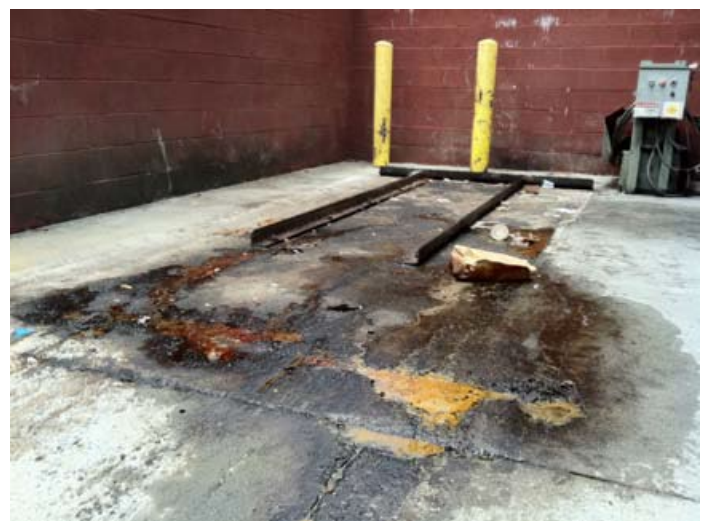
Figure B3-2 Leaking Dumpsters and Solid Waste Containers Can Be a Significant Source of Stormwater Pollution
