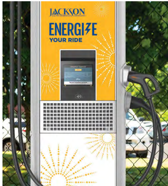
Public EV Charging Stations at Jackson EMC Offices
