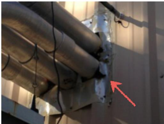
Photograph No. 4: EC-03-01 through 03: Pipes on East Wall Attached to Structure No Asbestos Detected
