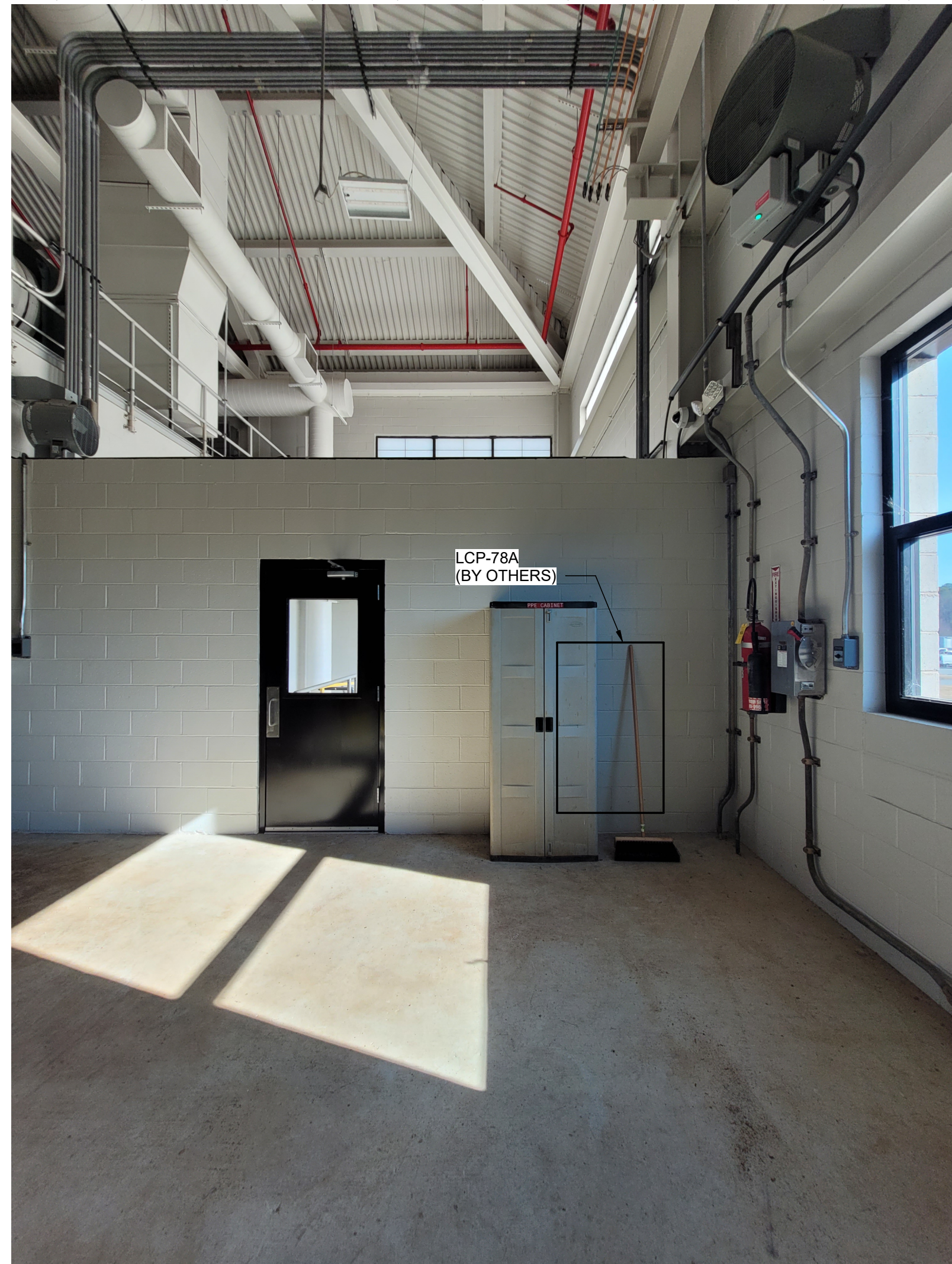
PANEL LCP 78A LOCATION - LIME AREA UPPER LEVEL
