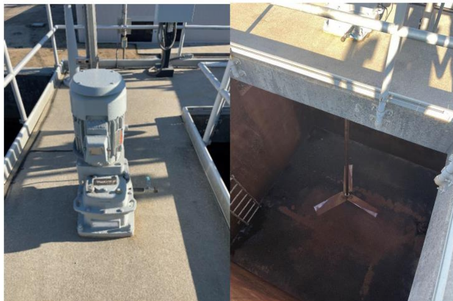
Figure 2 – Typical Existing Pre-Clarification Vertical Flocculator
