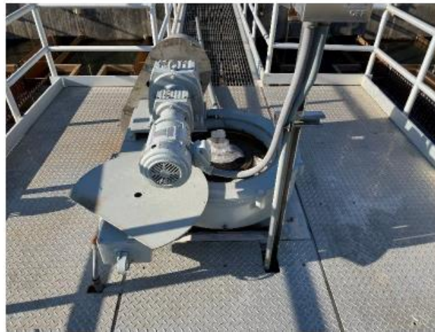
Figure 2 – Existing Pre-Clarification Basin Drive Unit
