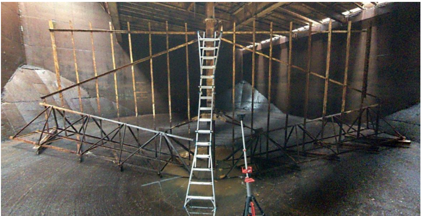
Photograph 4 – Pre-Clarification Basin Rake and Squeegees
