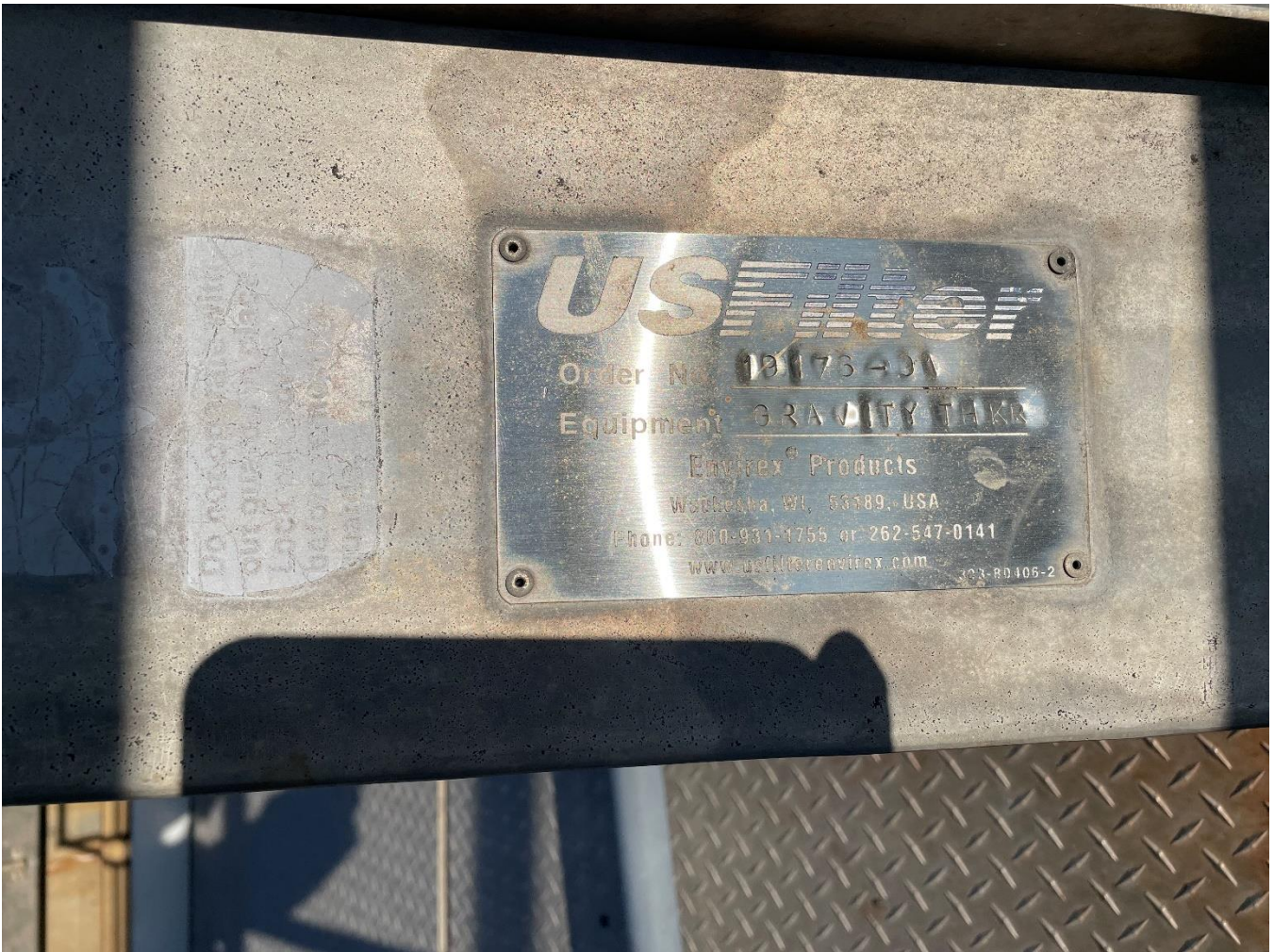
Photograph 6: Equipment Name Plate
