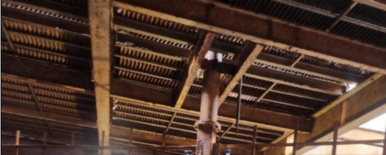
Photograph 5: Pre-Clarification Basin Torque Tube
