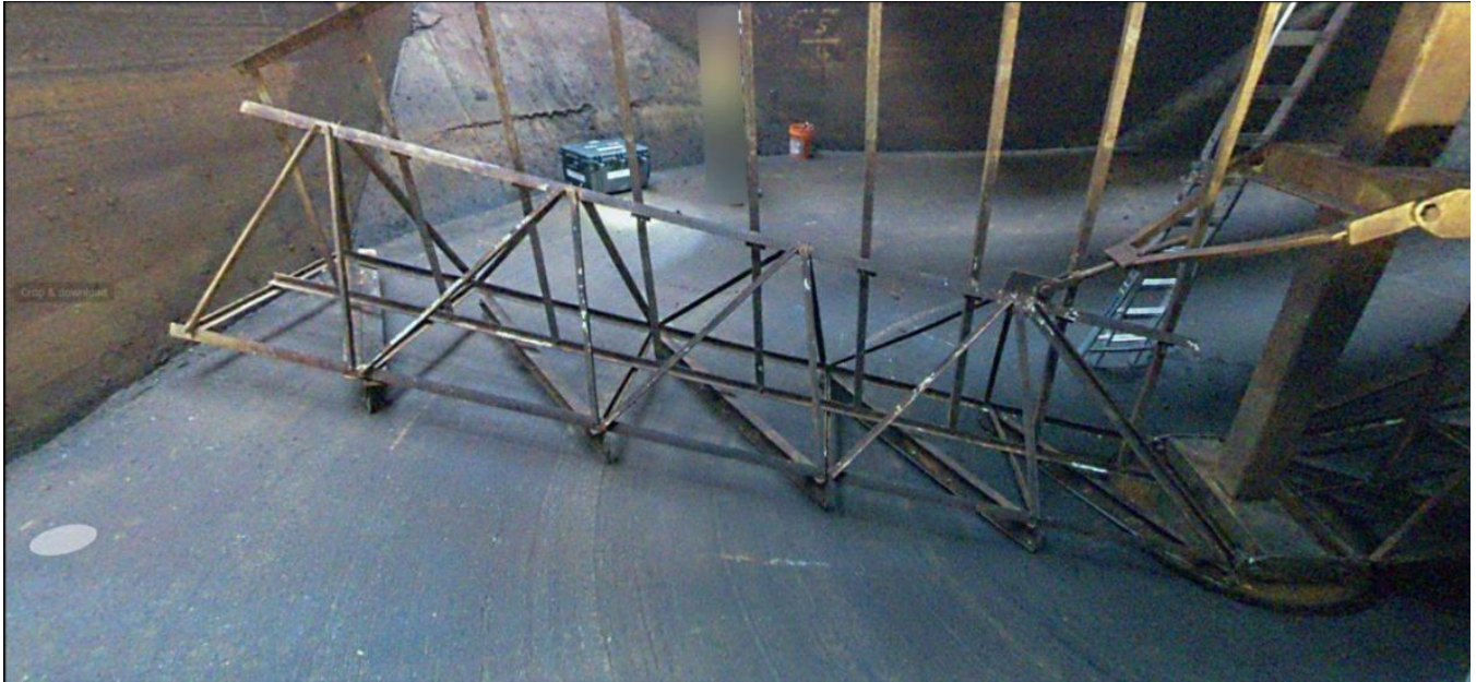
Photograph 3 – Pre-Clarification Basin Rake and Squeegees
