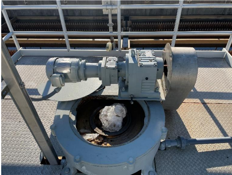
Photograph 1: Existing Drive Unit
