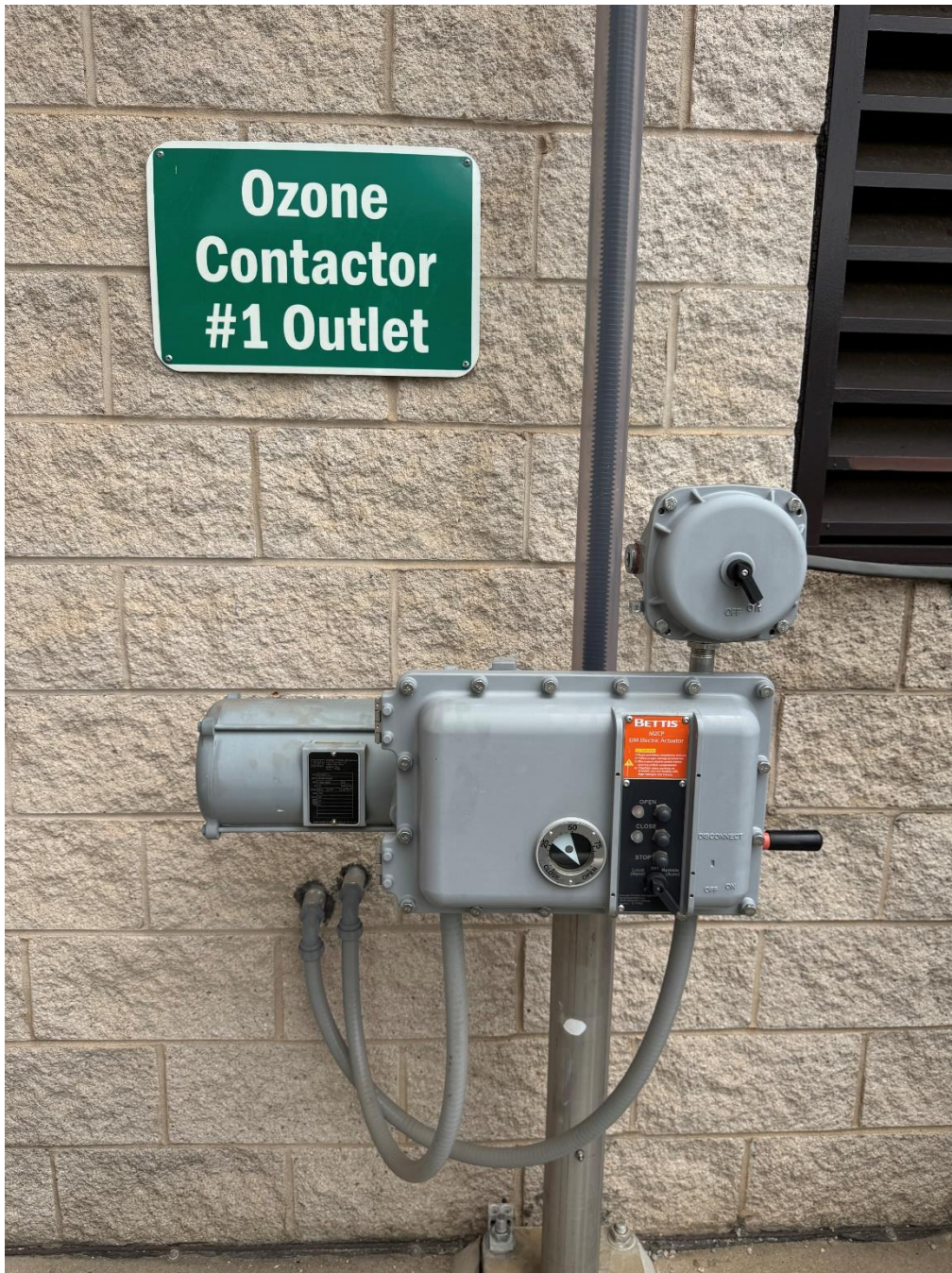
Photo 6: Typical Exterior Actuator Installation in Ozone Facility
