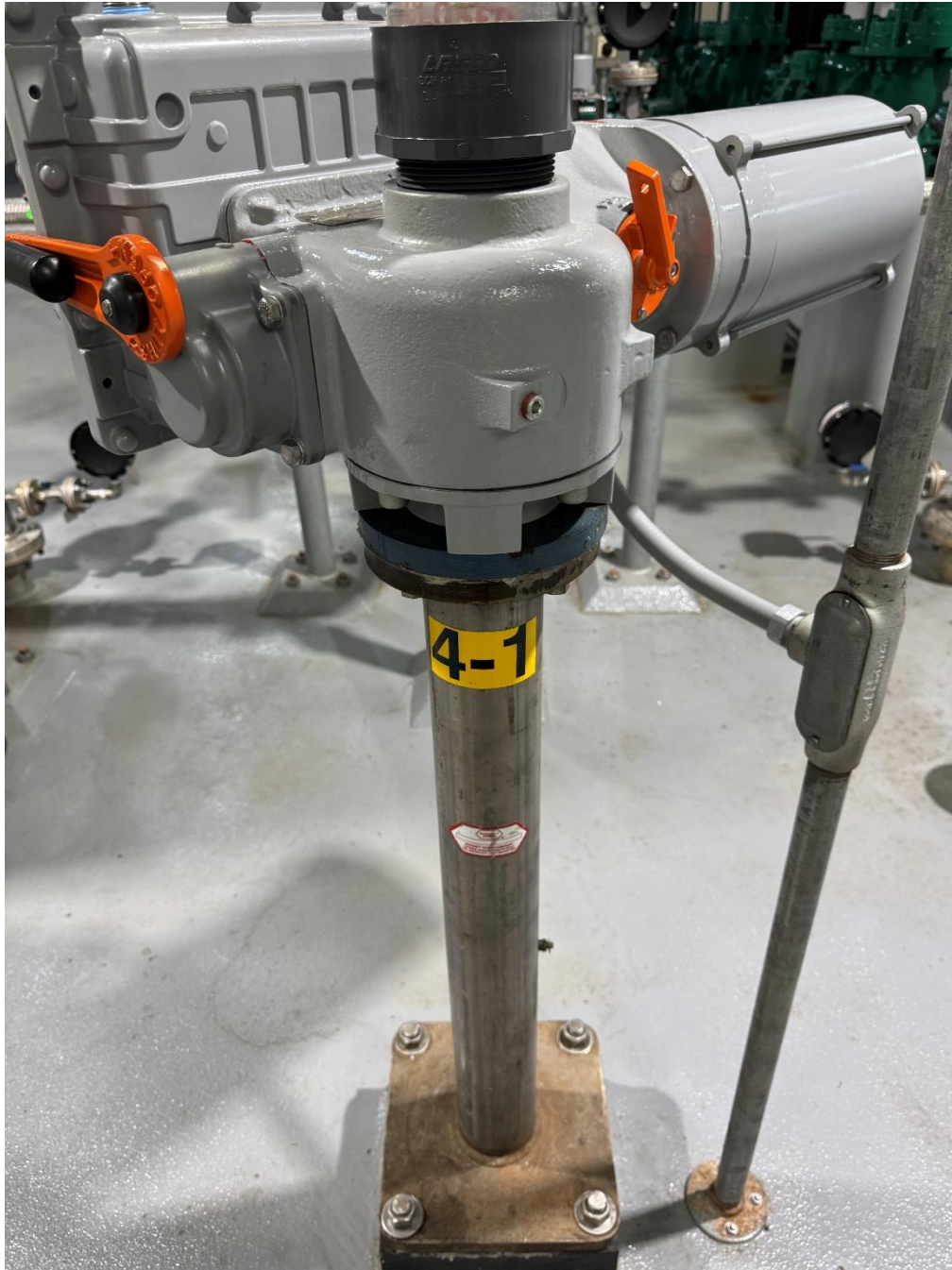
Photo 6: Typical Interior Actuator Installation in Ozone Facility
