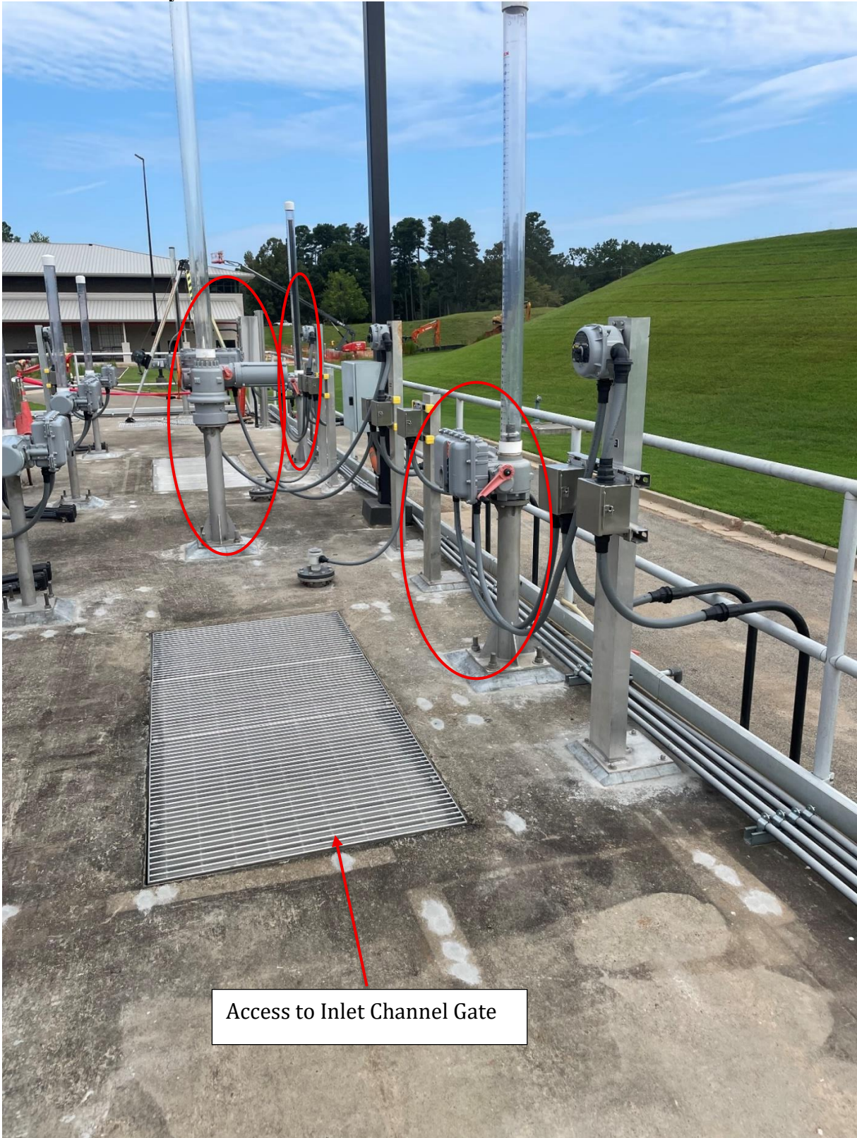
Photo 1: Gates and Operators on the Inlet Side of the Pre-Treatment Basin
