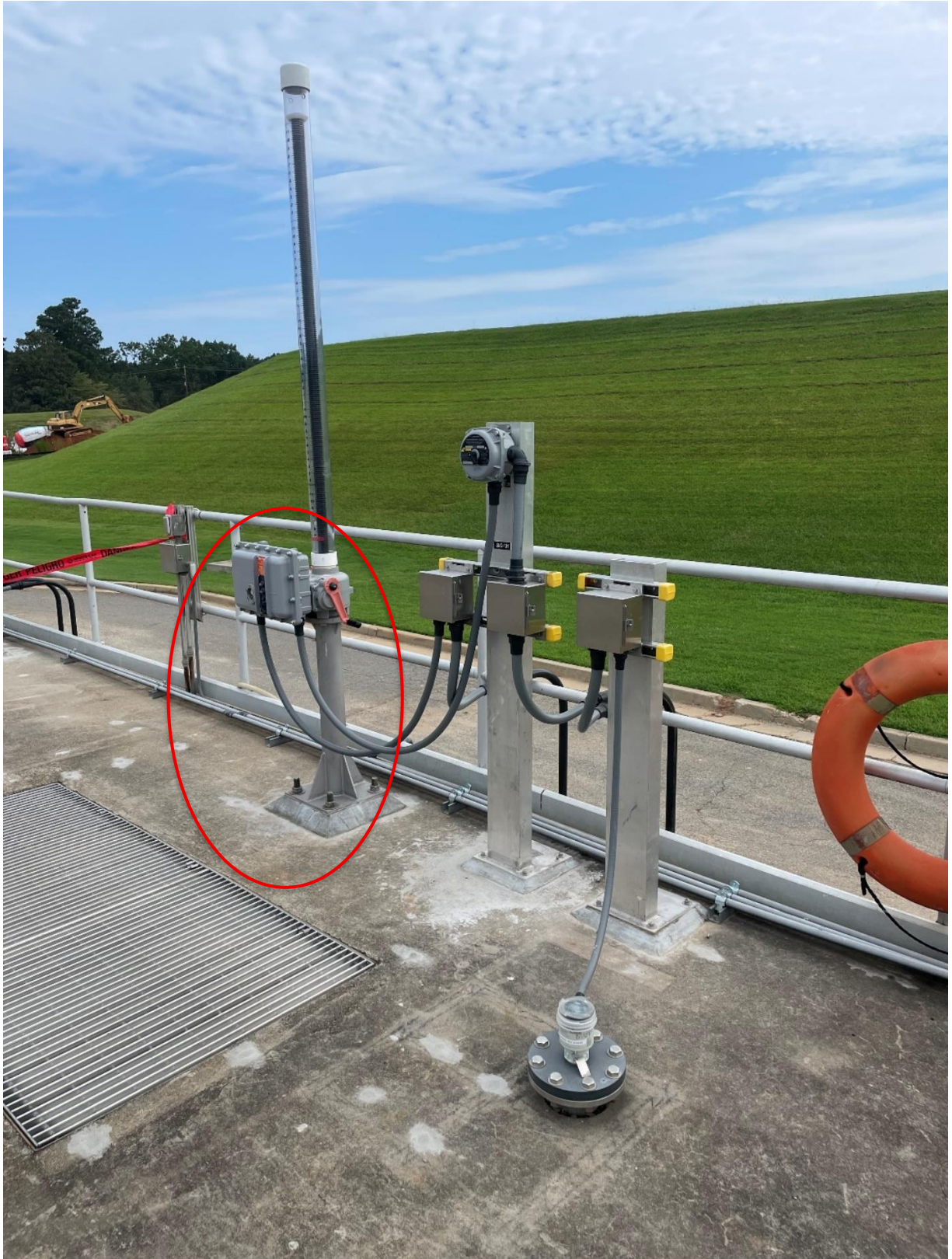
Photo 3: Inlet Gate Operator
